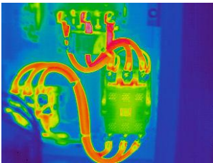
Overheating motor contactor
